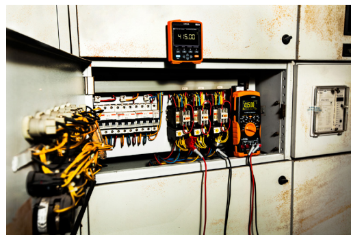
Figure 3. Monitoring handheld meter readings via the U1115A remote logging display
